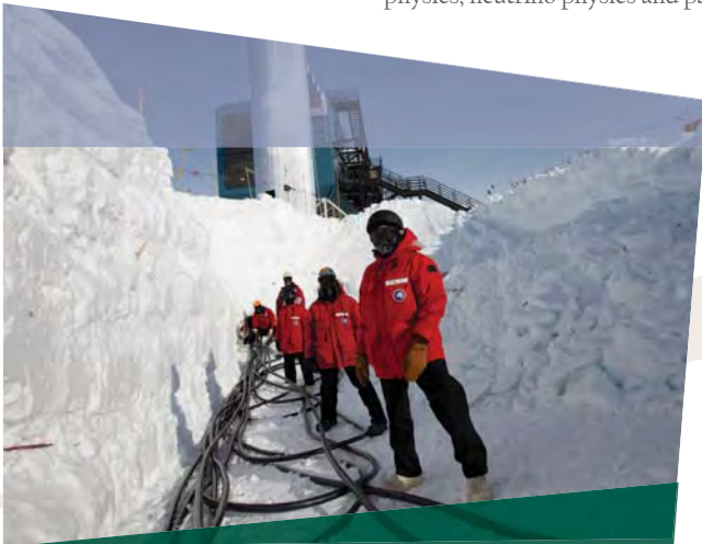
Laying cables for the ICECUBE detectors that are embedded in several cubic kilometers of ice at the South Pole.
